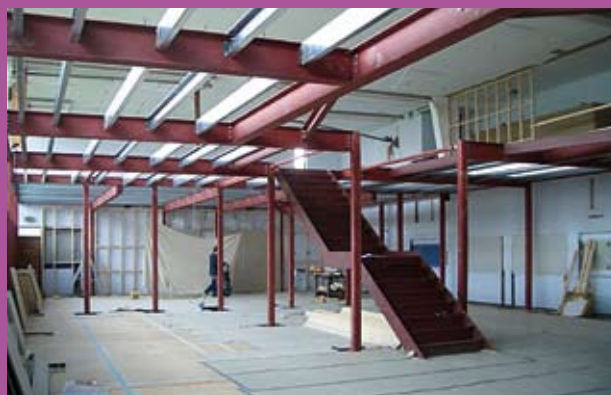
2. The creation of a mezzanine floor was an obvious solution to maximising space, although it did lead to complications; minimum floor-to-ceiling heights were only just manageable
